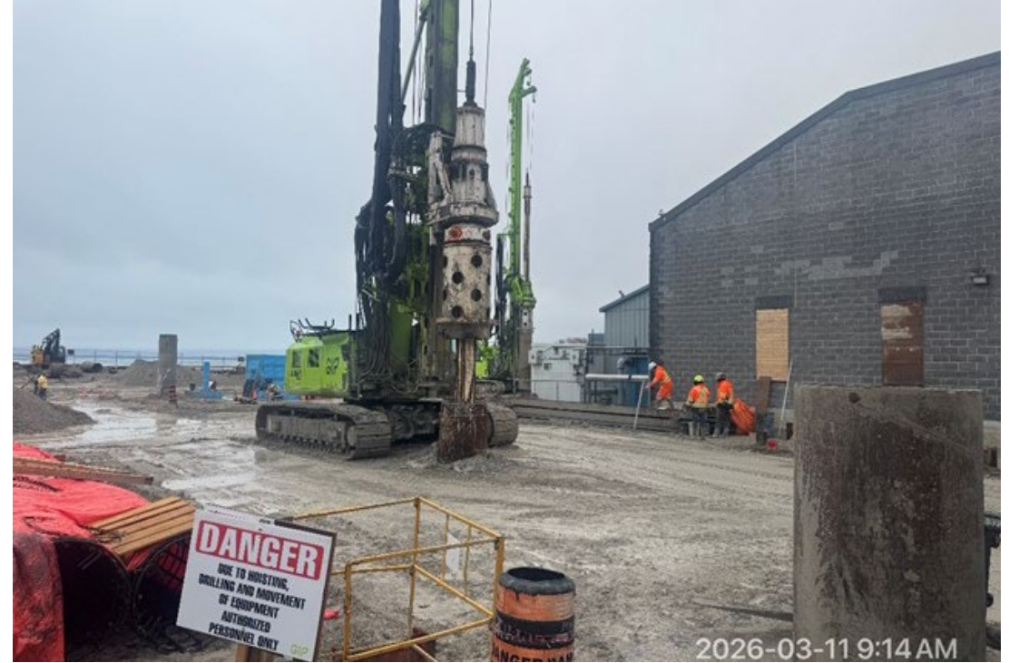
Installation of a caisson for the new onsite sewage pumping station valve chamber
