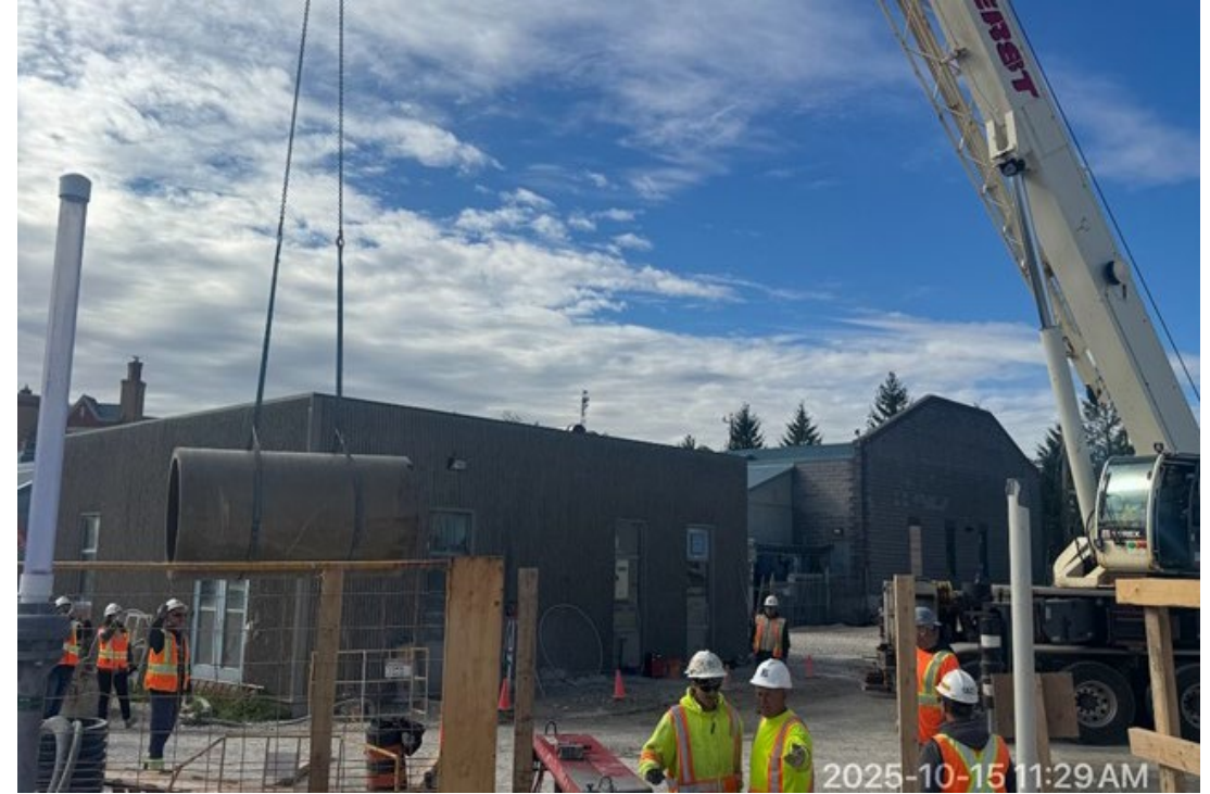
Cut and removed a portion of the of the 1050mm intake pipe from Intake No. 1 Chamber.
