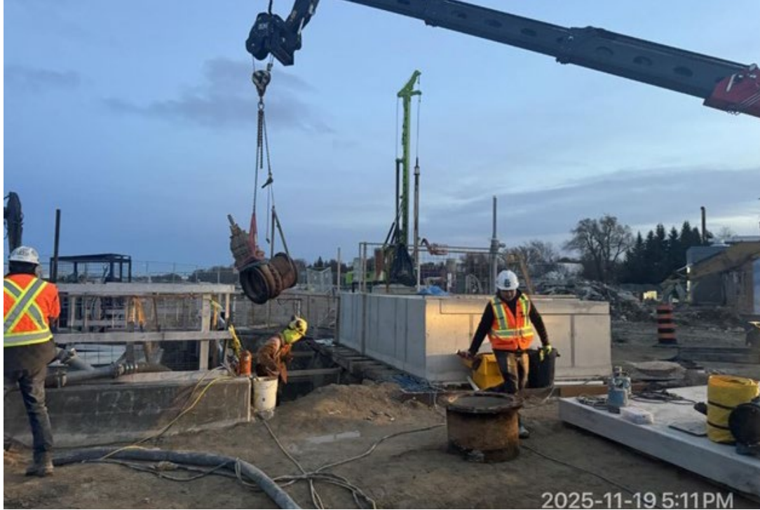
Cut and removed the east bypass gate valve from Intake No. 1 Bypass Chamber.
