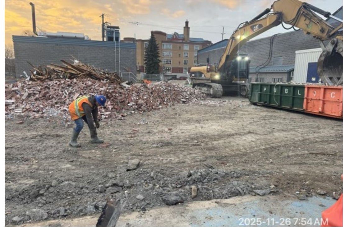
Demolished the existing Raw Water Building and Industrial Pumping Station (IPS) and removed the waste from site.
