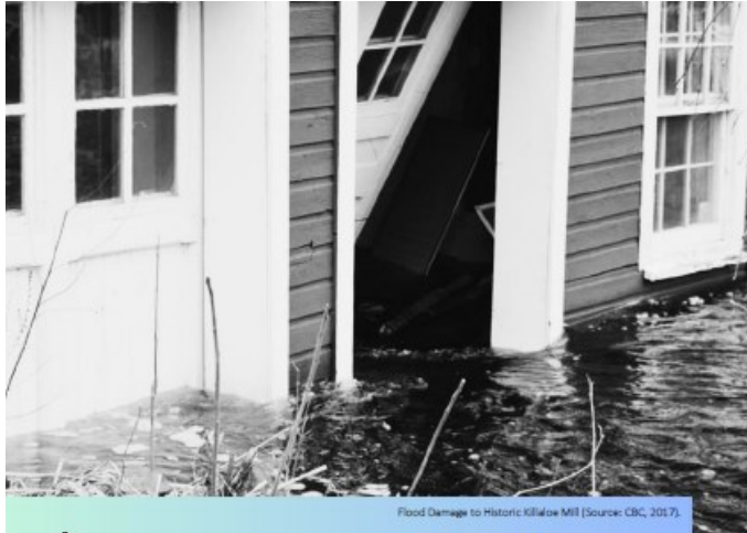
Flood Damage to Historic Killaroe Mill (Source: CBC, 2017).
