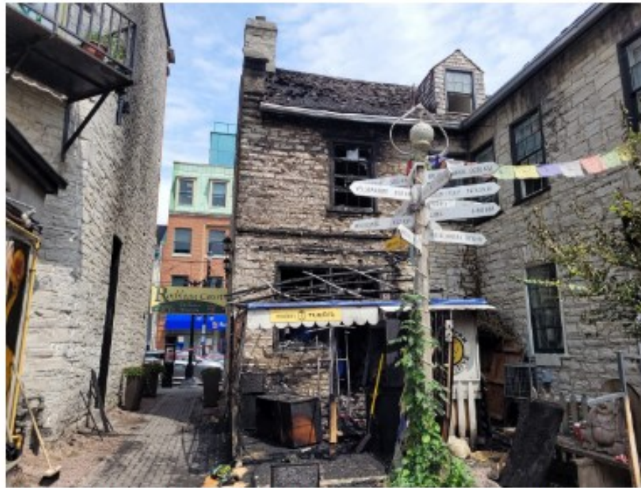
The damages visible on the courtyard area behind Modern Primitive following a fire that broke out on Thursday, Aug. 4, 2022.
