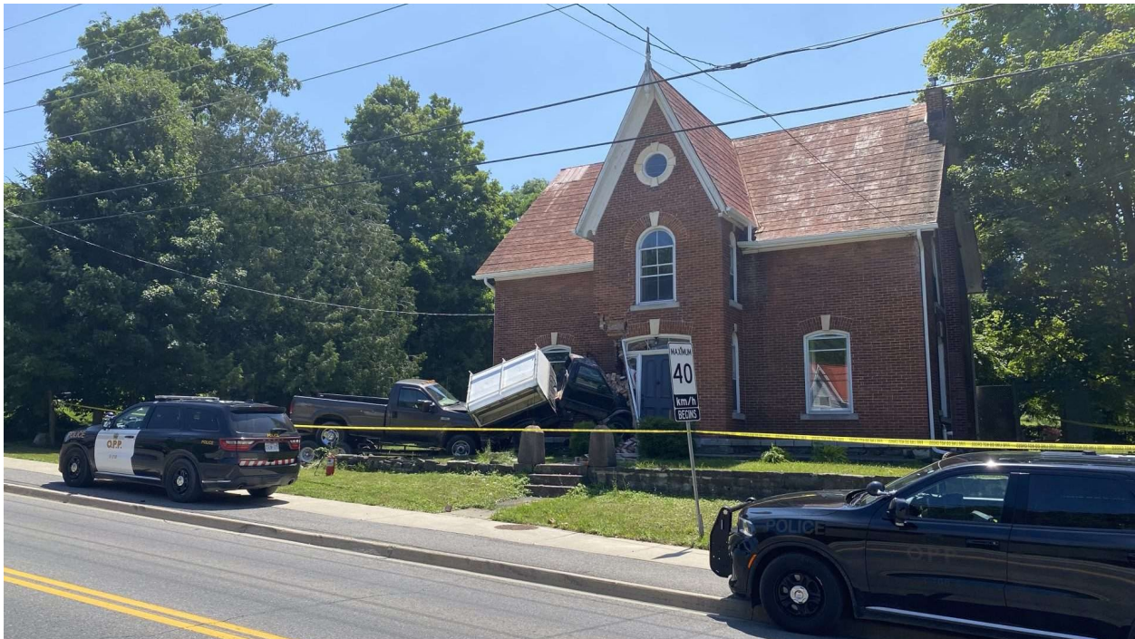
Figure 29 - Damage caused to a building in Sydenham, Ontario, due to a vehicle collision (Source: Vilela, 2023)
